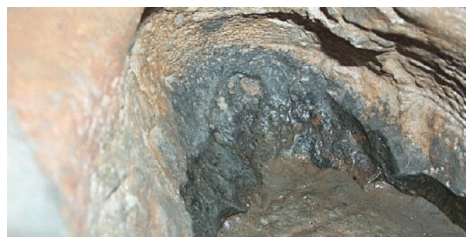
Davis-Besse corrosion | NRC
